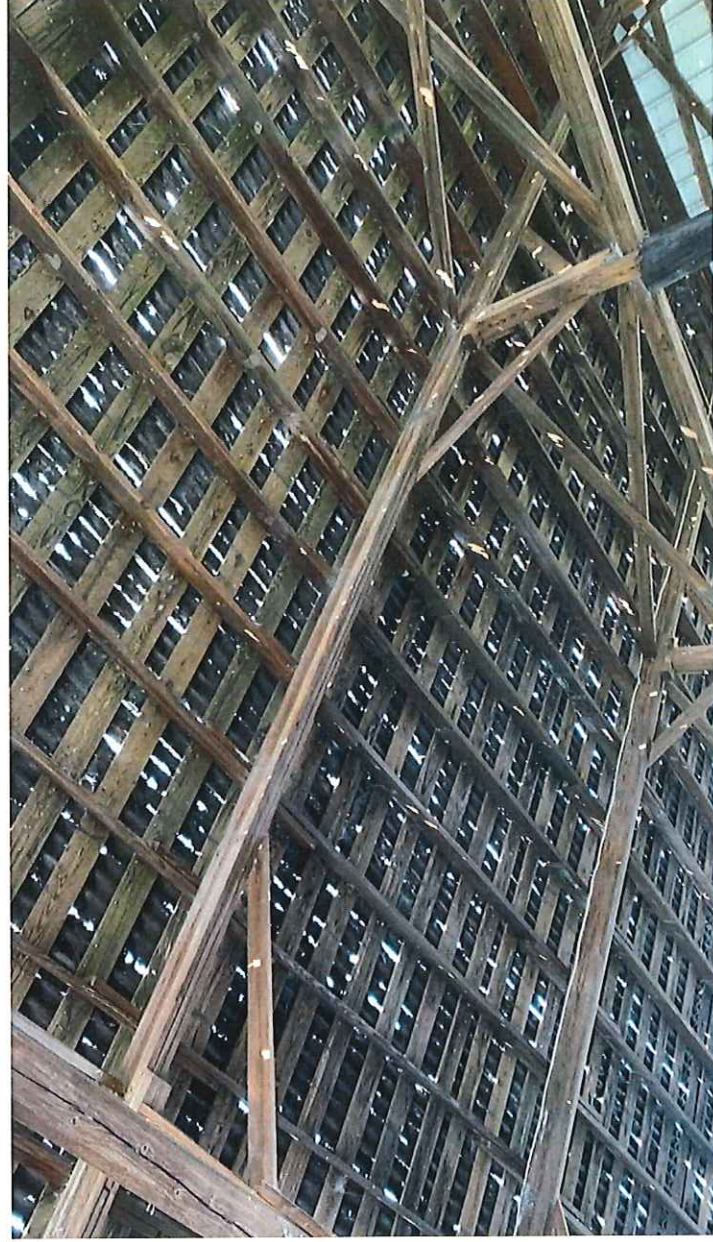
Image: Thousands of holes are clearly visible in the roof deck on L-Dock. The failed roof system has led to severe degradation of structural elements.
